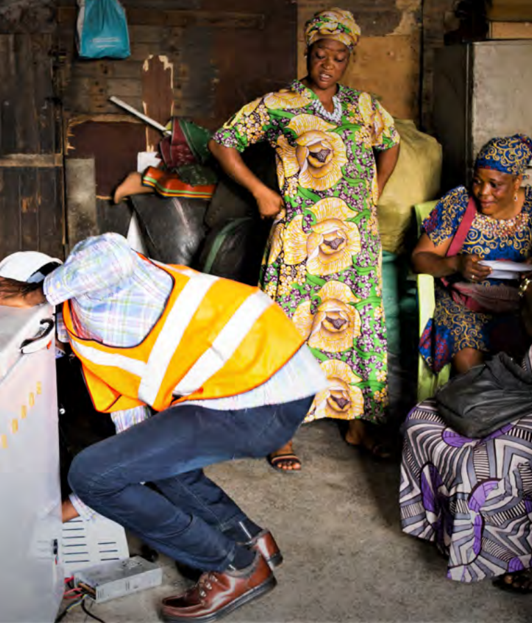
Fish traders watch with excitement as Koolhome solar freezer is installed at Ijora Market in Lagos, Nigeria
