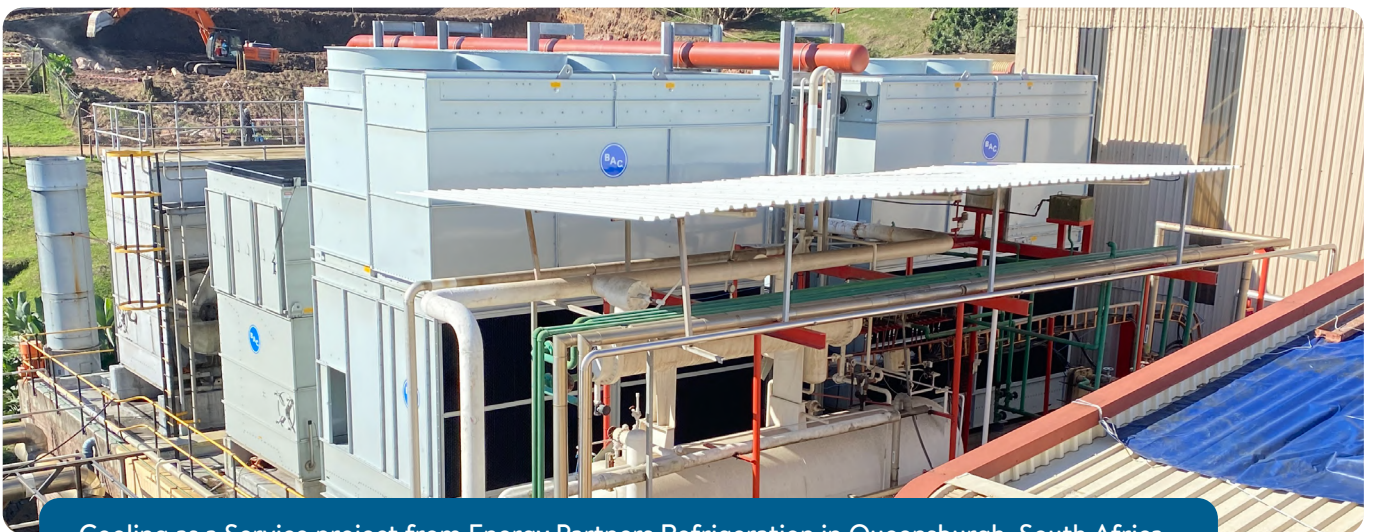
Cooling as a Service project from Energy Partners Refrigeration in Queensburgh, South Africa
