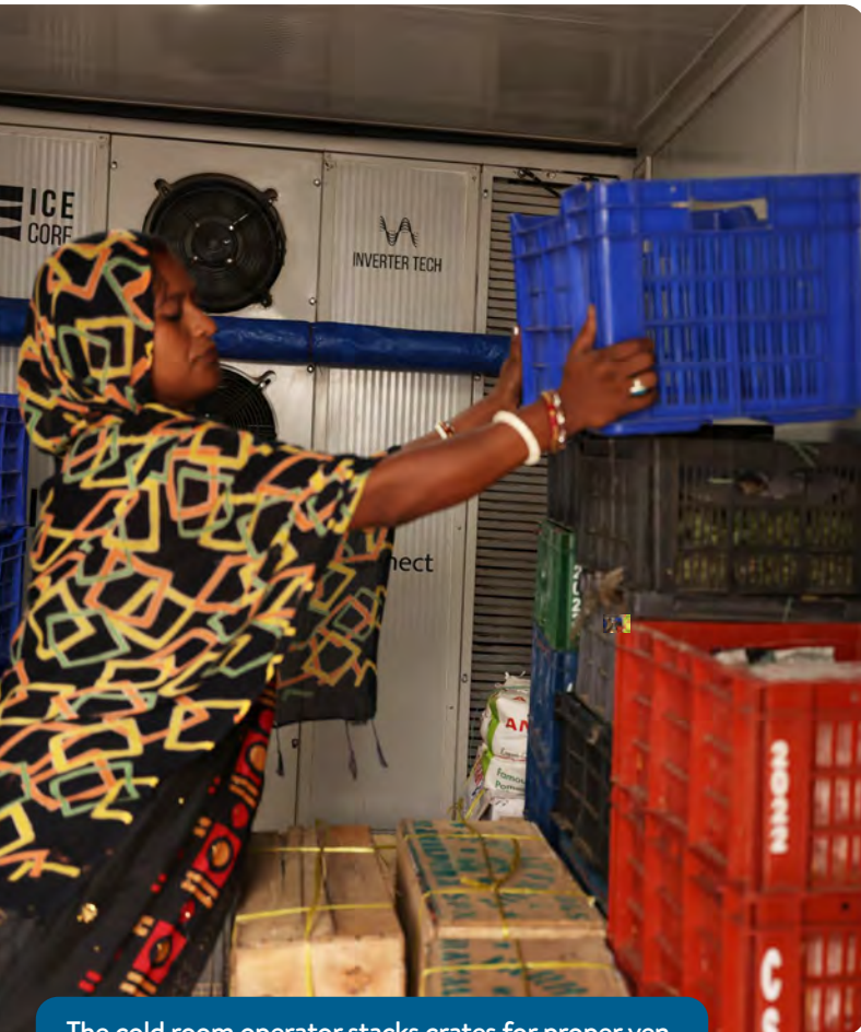
The cold room operator stacks crates for proper ventilation of crops at Oorja's cold room in Bihar, India.
